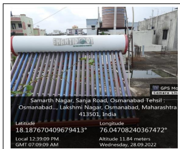
Solar Water Heater
